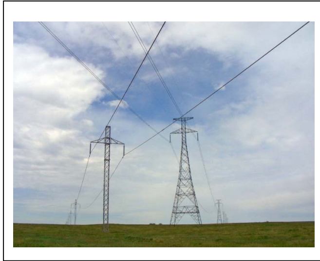
Fig. 12: HVDC allow power transport over long distances with reduced losses. Only two cables are necessary contrary to usual AC lines (3 cables).
