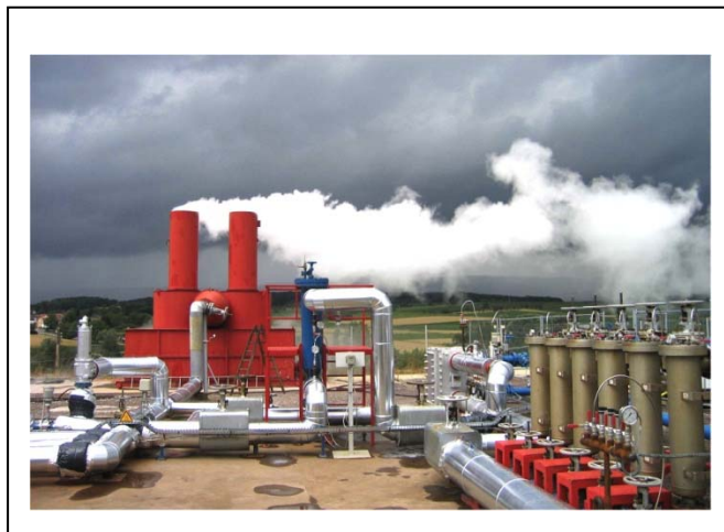
Fig. 10: A prototype (2 MW) geothermal power plant running at Soultz (France).
