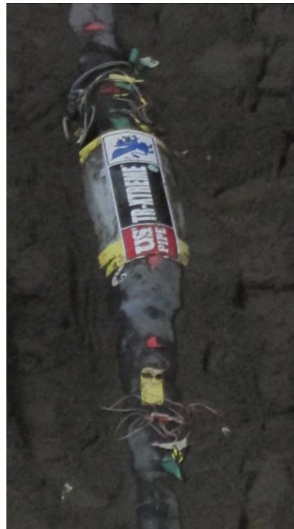
b) Failure at South Joint
