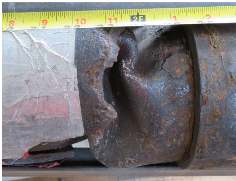
Figure 6.10. DC2 Deformed and Buckled Lining
