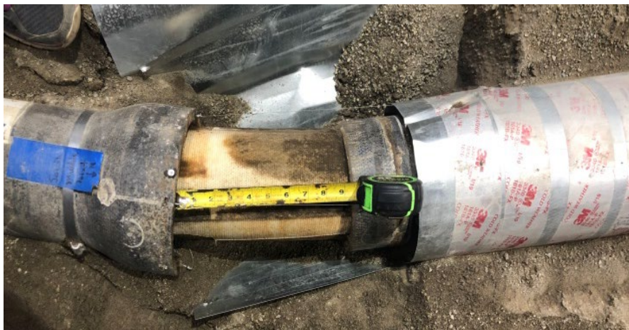
Figure 9.27. Deformation at South Middle Joint
