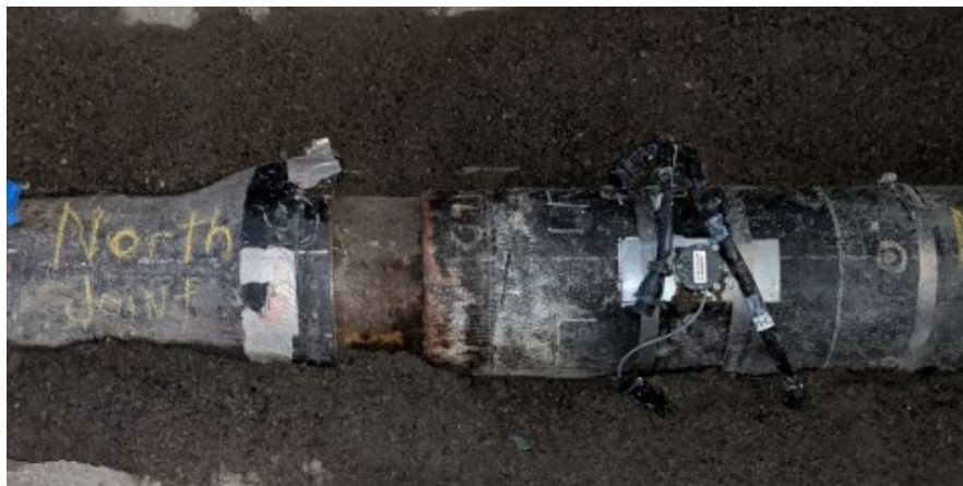
Figure 9.25. Deformation at North Joint
