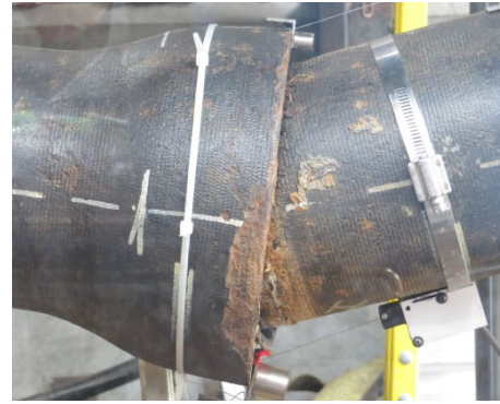
b) Corroded Pipe Joint
