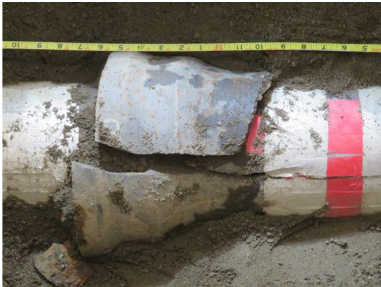
Figure 6.9. DC2 Fractured CI Bell
