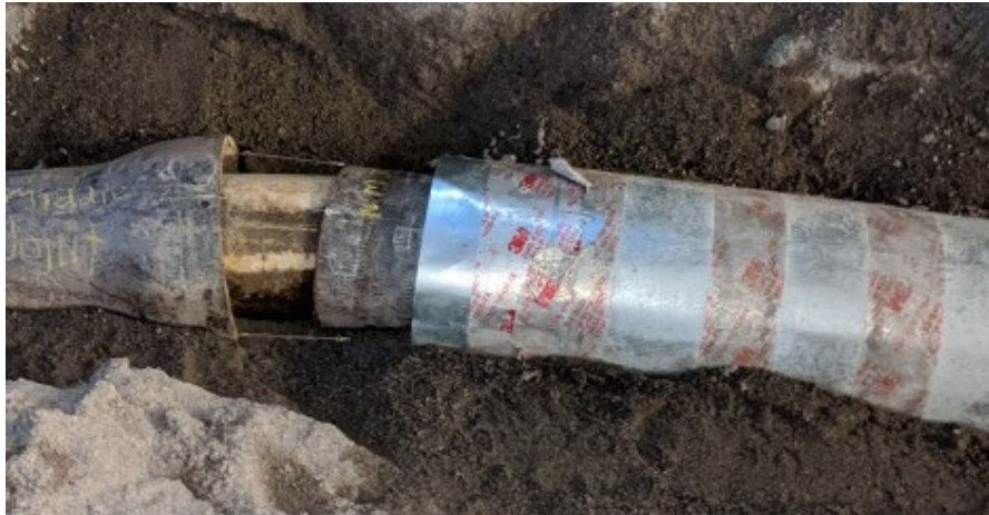
Figure 9.26. Deformation at North Middle Joint
