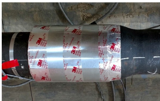
Figure 9.2. Joint Instrumentation Protective Shielding
