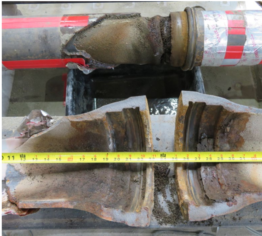
Figure 6.15. DC 4 Fractured CI Bell and Deformed Aqua-Pipe Lining
