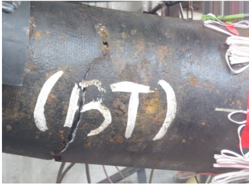
a) Corroded Pipe Barrel
