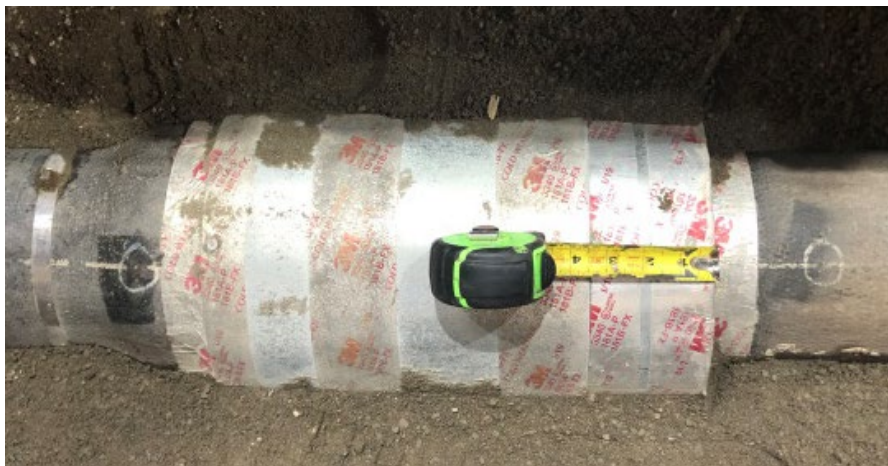
Figure 9.28. Deformation at South Joint
