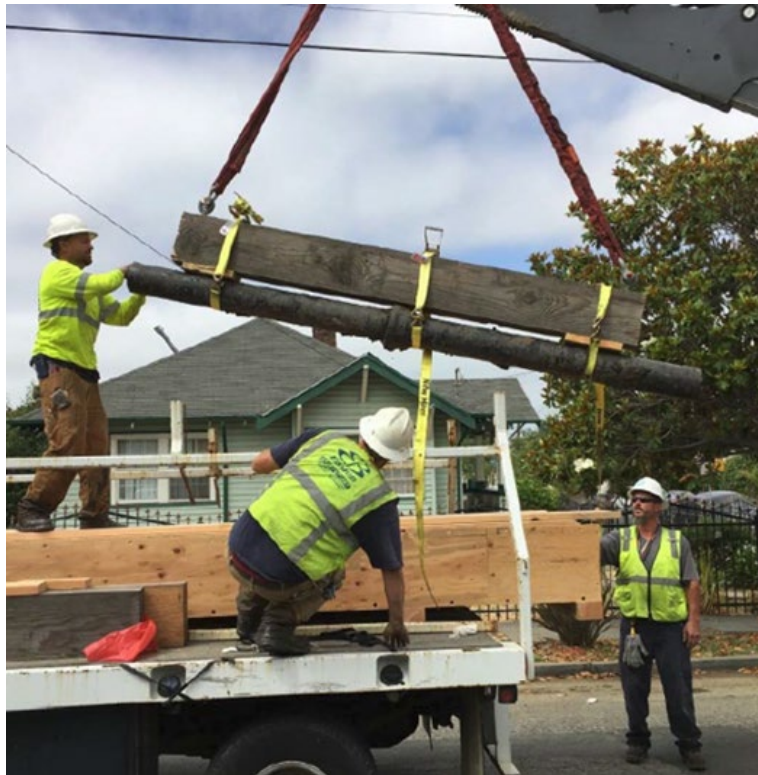
Figure 6.3. EBMUD Retrieval of a Jointed Pipe Specimen
