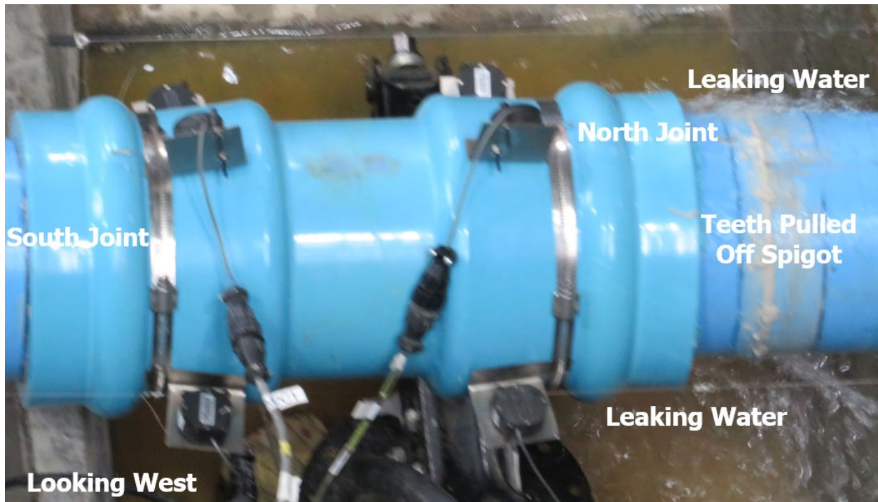
Figure 3.9 Photo of Leaking iPVC™ Fitting for Second Tension Test
