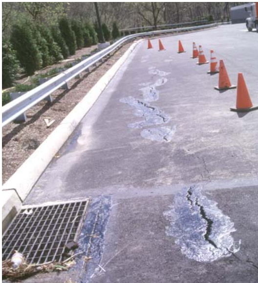
Figure 30. Cracks on crest
