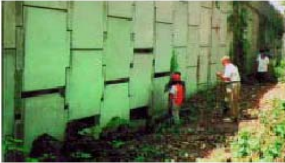
Figure 26. Settlement from pipe leakage
