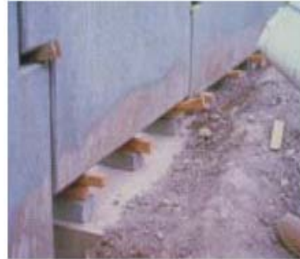
Figure 7. Improper leveling pad
