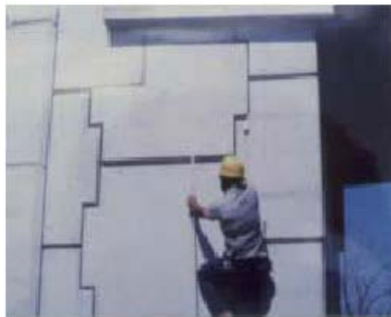
Figure 24. Joints opening from settlement
