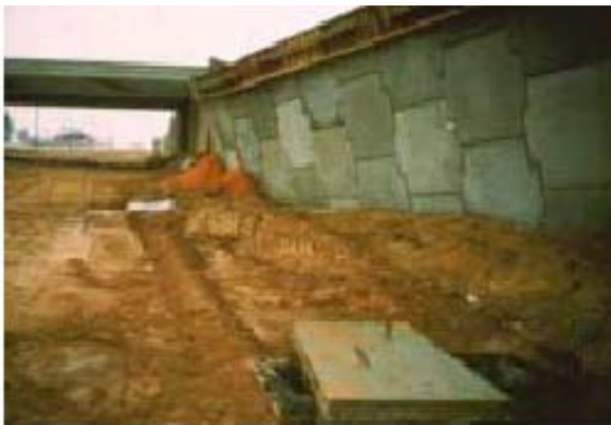
Figure 25. Failure from exterior excavation
