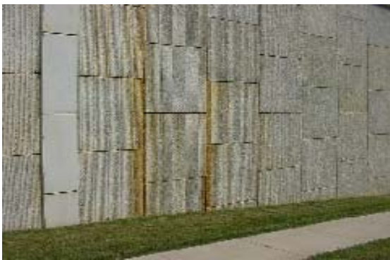
Figure 27. Staining on panels
