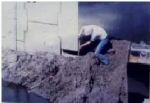
Figure 23. Settlement from excavation
