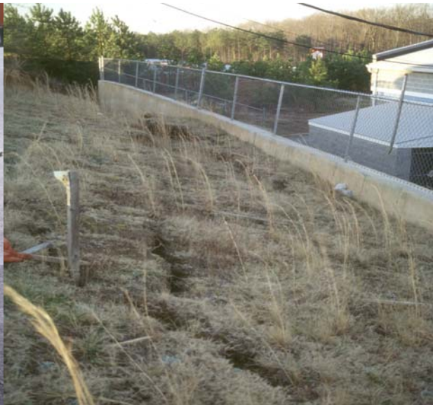
Figure 31. Tension cracks in backfill
