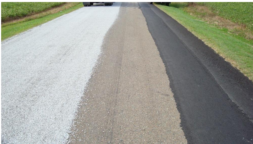
Figure 3 Finished chip seal on the left, oxidized pavement in the center and hot mix widening on the right, both ready to receive chip seal
