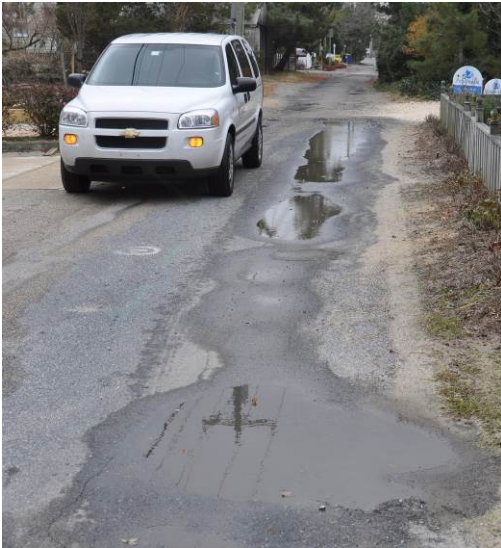
Right of way, geometry, drainage, and roadside land use can be challenging for local roads.
