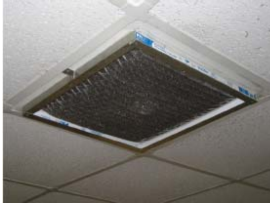
Figure 6. Add-on Ceiling Filters Showing Dirty Element, Richards & Robbins Laboratories. Source: (2rw Consultants Inc., 2004)
