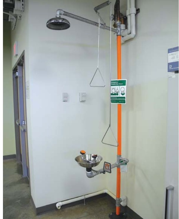
Figure 2. Accessible Emergency Shower and Eyewash.
