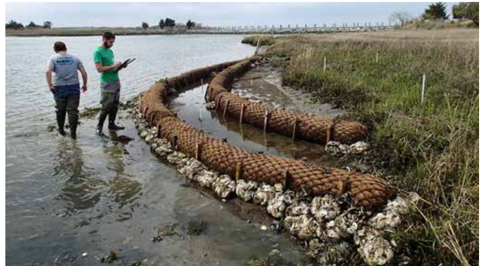
Figure 7: Use of coir logs and oyster bags by DNREC living shoreline site, via DNREC Living Shoreline Committee.
